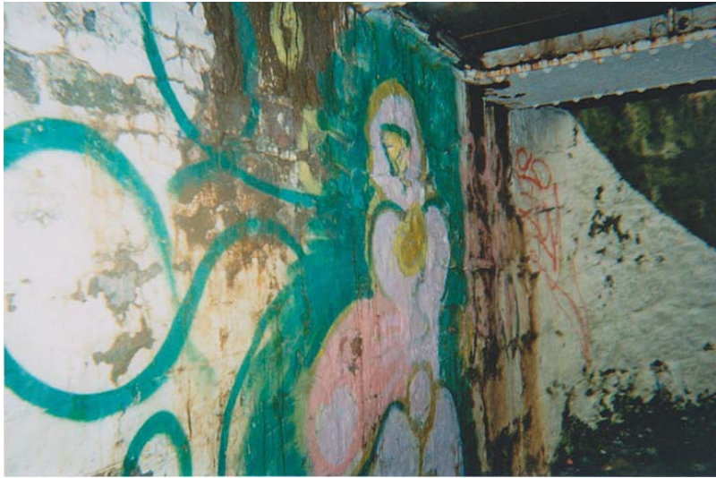
Figure 4. 'Graffiti under a bridge which is bang out of order ... look it's just disgusting, look at that - it's actually just inappropriate and it's making us look disgusting n like a minky place. and it makes me feel like a mink ... it makes me feel depressed because it's actually bang out of order.' Notes: Photograph and quote - Participant 2, Category - Perceived investment, Theme - Disinvestment.
