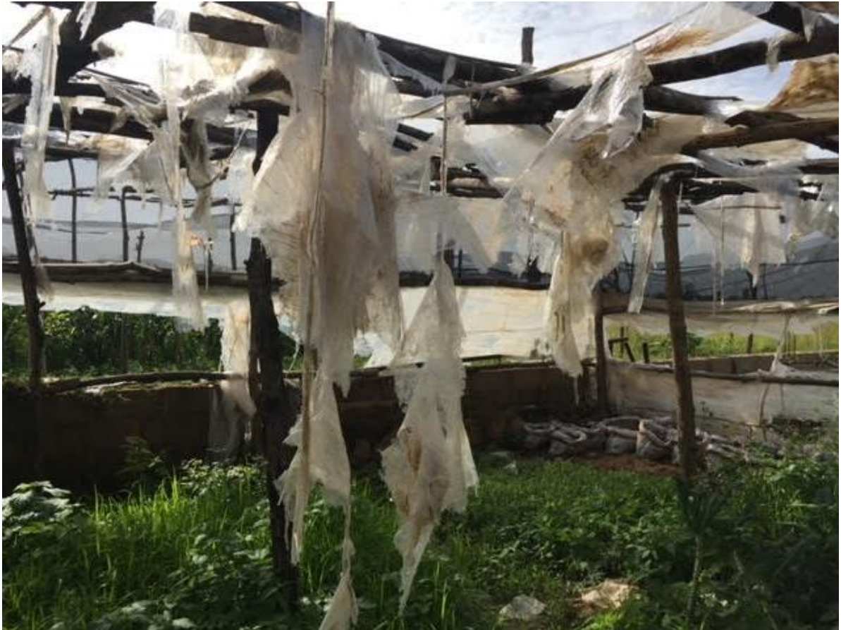
Figure 6.10 Poorly constructed Greenhouse
