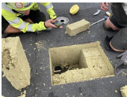
Figur11. Measurement on roof with a wood block under the sensor - by Woodsence
