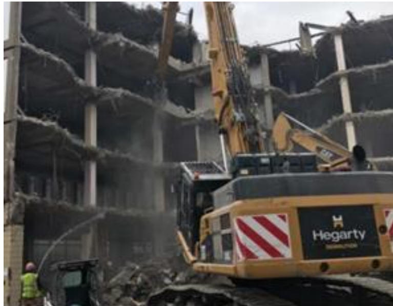
Figure 5. Deconstruction of Oisín House with the goal of “Zero Waste to Landfill”.
