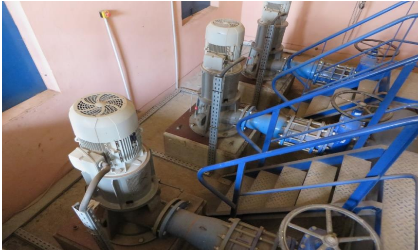
Figure 4-4: Broken-Down Water Pumps Supplied by a Previous Project in Southern Togo
