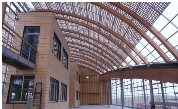
Figure 5. Skylight with monocrystalline PV modules [65].
