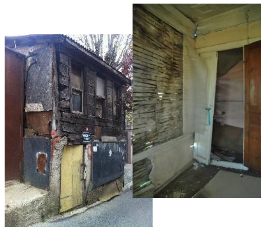
Figure 3. A typical ruined Bosphorus mansion, exterior view and the condition of the external walls from inside [author archive].
