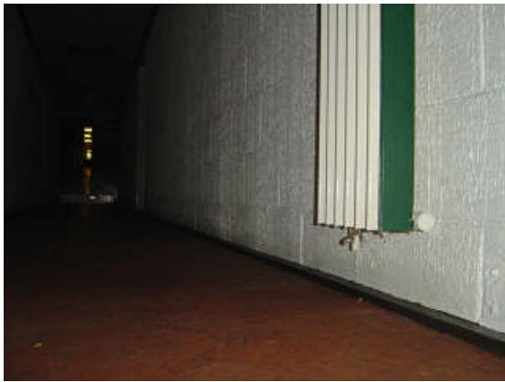
Figure 1. 6 A radiator in the corridor environment
