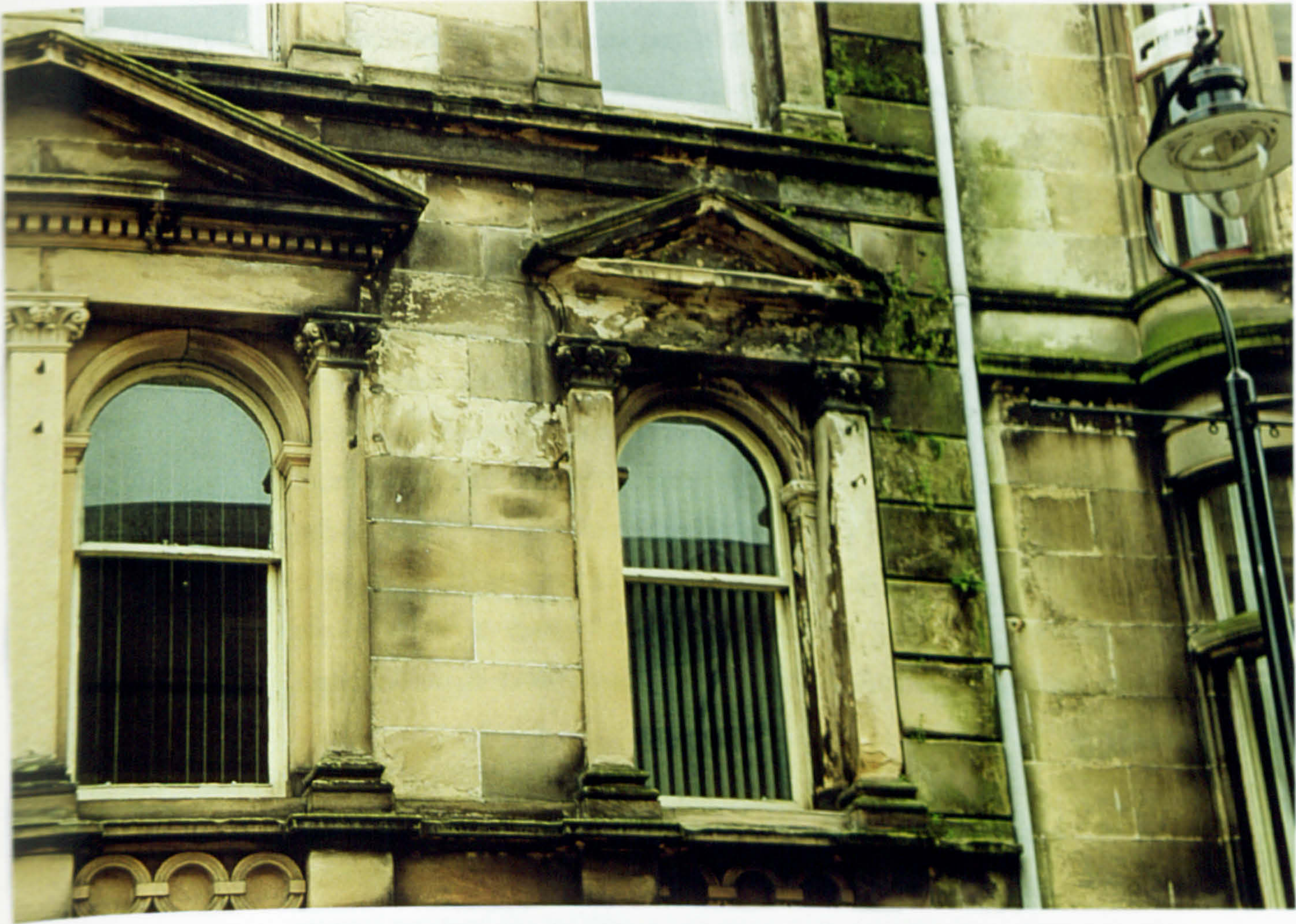
Figure 7.8 - Spalling and algal growth on neighbouring property
