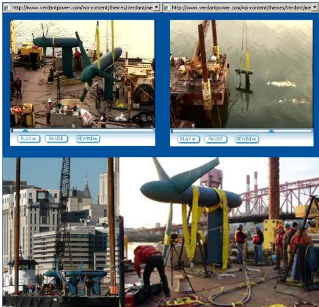
Figure 2.43: New York East River installation (43)
