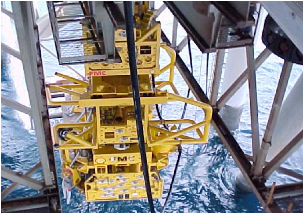
Figure 2.29: Subsea tree, LRP and EDP below rig floor being deployed (20)
