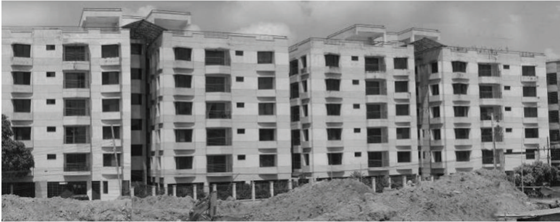
FIGURE 2: Increasing density and expanding footprint are supported by weak building bilaws (Photo credit: Quazi M Mahtab-uz-Zaman, 2006).
