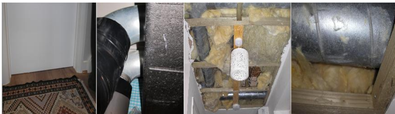
Figure 3. Mechanical ventilation system problems.
