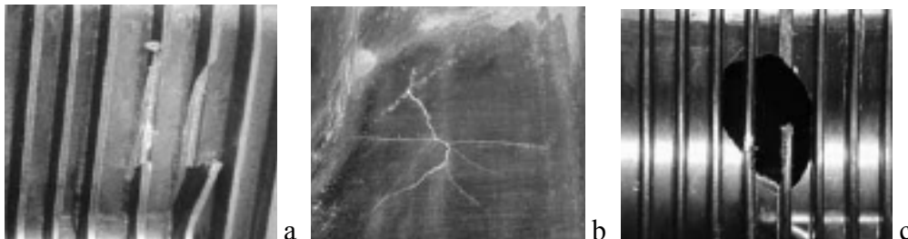
Figure 7. Damage types that can result after an impact. Broken ribs (a), Interior cracks (b), Perforation (c).
