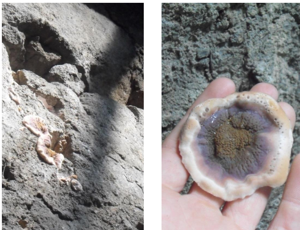
Figure 7-6 Dry rot growth on a party granite wall behind the lath and plaster. The wall had been exposed for treatment and all the affected timber removed.
