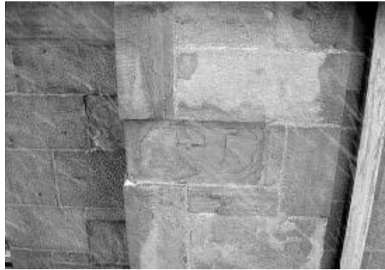
Figure 2-22 View of stone masonry deterioration from freeze-thaw following the installation of thermal insulation on the building interior (Carpenter et al. 2010)
