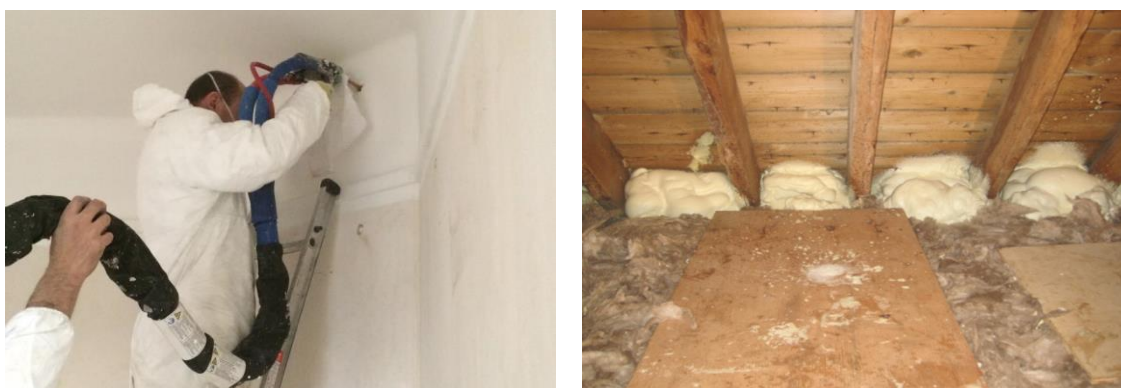
Figure 2-9 PUR foam application, (left) cavity injection (Historic Scotland 2015) and (right) foam at the eave level (courtesy of Dr Bennadji)
