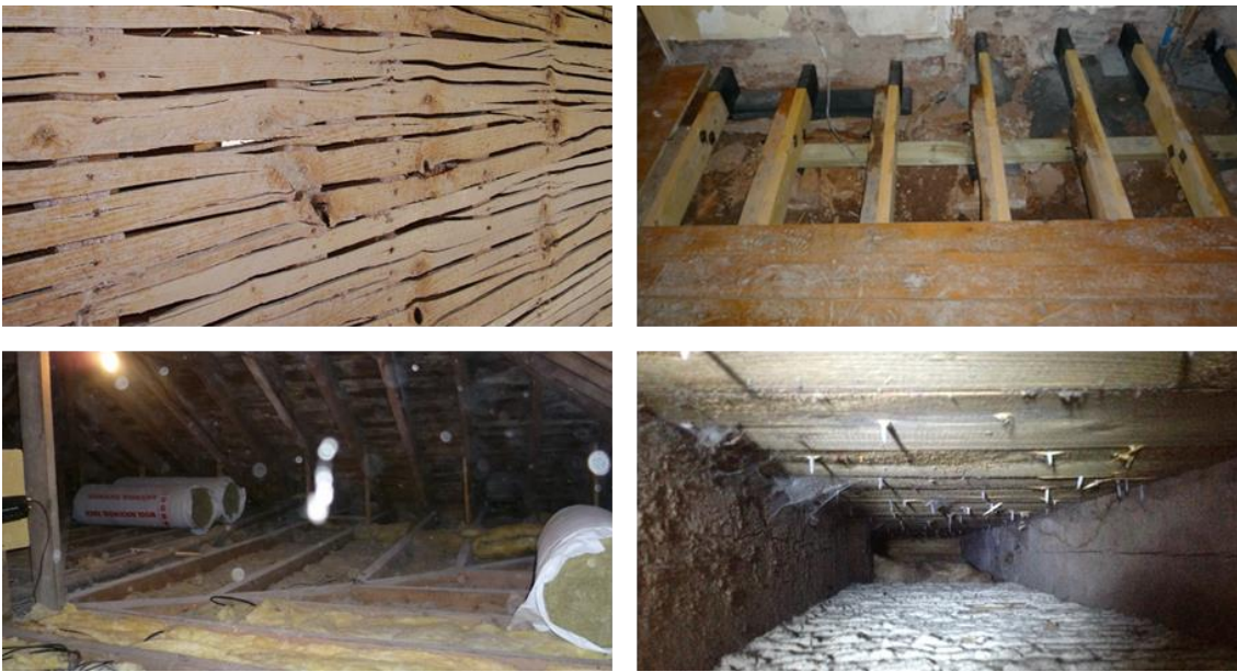
Figure 2-6 Original lath, suspended timber floor, loft insulation and coombes between roof and lath & plaster
