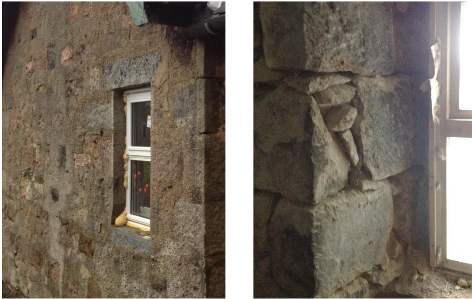
Figure 7-4 Kincardine O'Neill. Example of granite wall built using (a) rich mortar on the exterior and (b) a lean mortar in the core of the wall.
