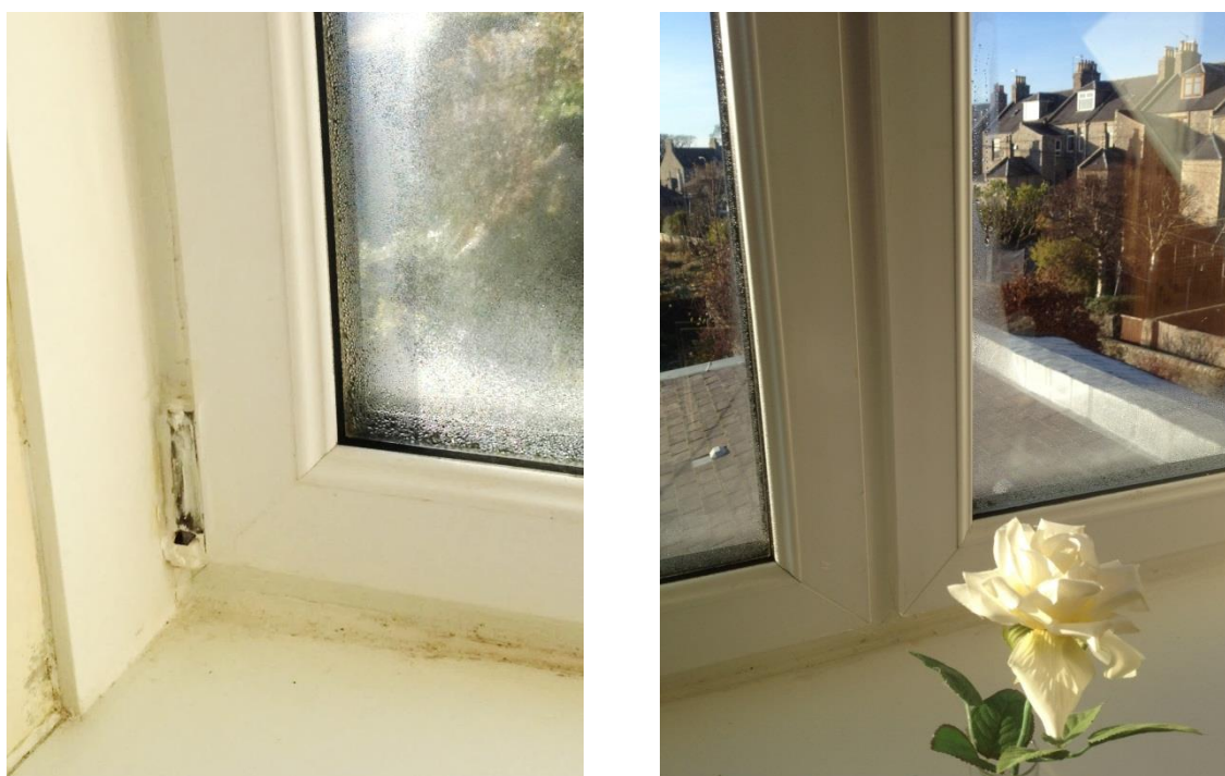
Figure 5-3 Case 16. Window frame was sealed up with a silicone gun.
