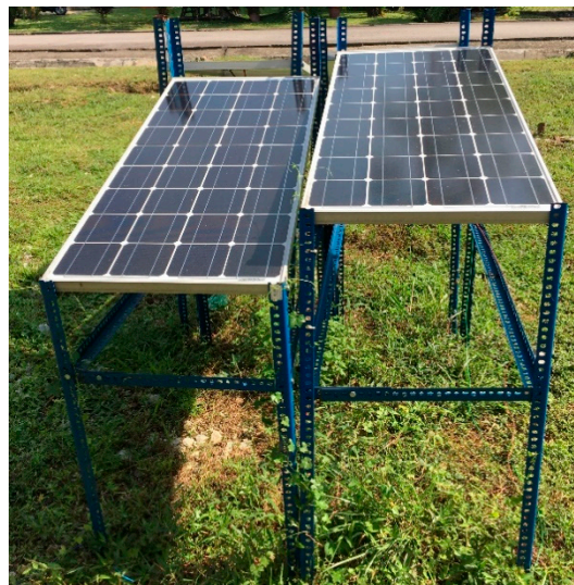
Figure 4. The side view of the PV panel arrangement at the G3 building in UTM, KL.
