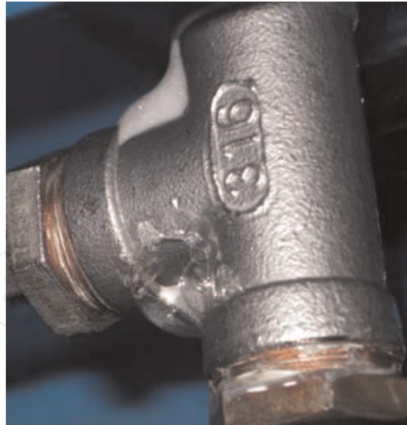
Figure 22. Source of leakage identified after on-site inspection.
