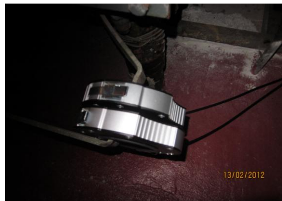
Figure 6 HFCT connection at the substation earth
