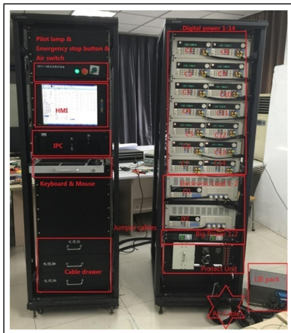
Figure 8. The battery maintenance and testing system (BMTS) for the maintenance of lithium-ion battery (LIB) packs.
